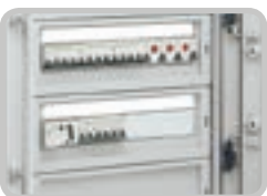
Detail from the circuit-marking system.
